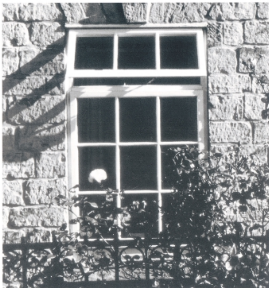
Modern wood replacements for traditional sash windows can be just as inappropriate as plastic or aluminium substitutes
