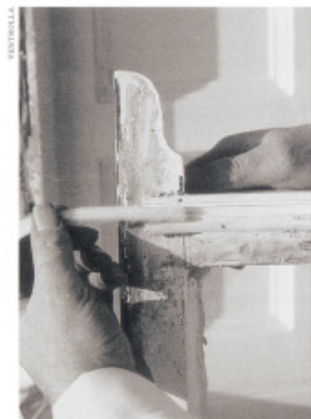
Reversible upgrading: inserting a brush weatherstrip into the meeting rail of a sash frame
