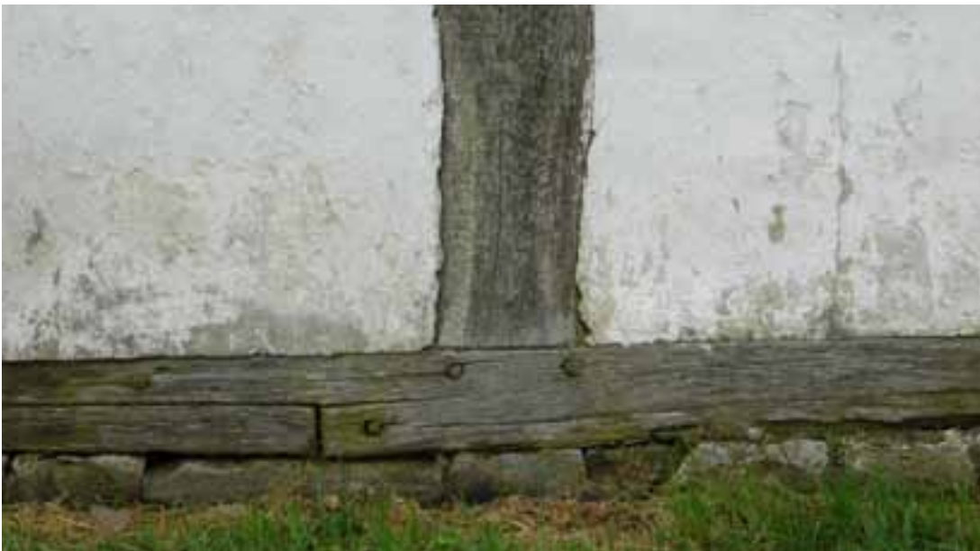
05 The most vulnerable part of the timer frame to damp is the lowest horizontal timber the sill beam or sole plate as this is the timber nearest the damp ground. © EH/David Pickles
