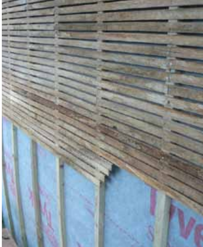
13 Timber laths being fixed externally over a vapour permeable membrane . © Oxley conservation
