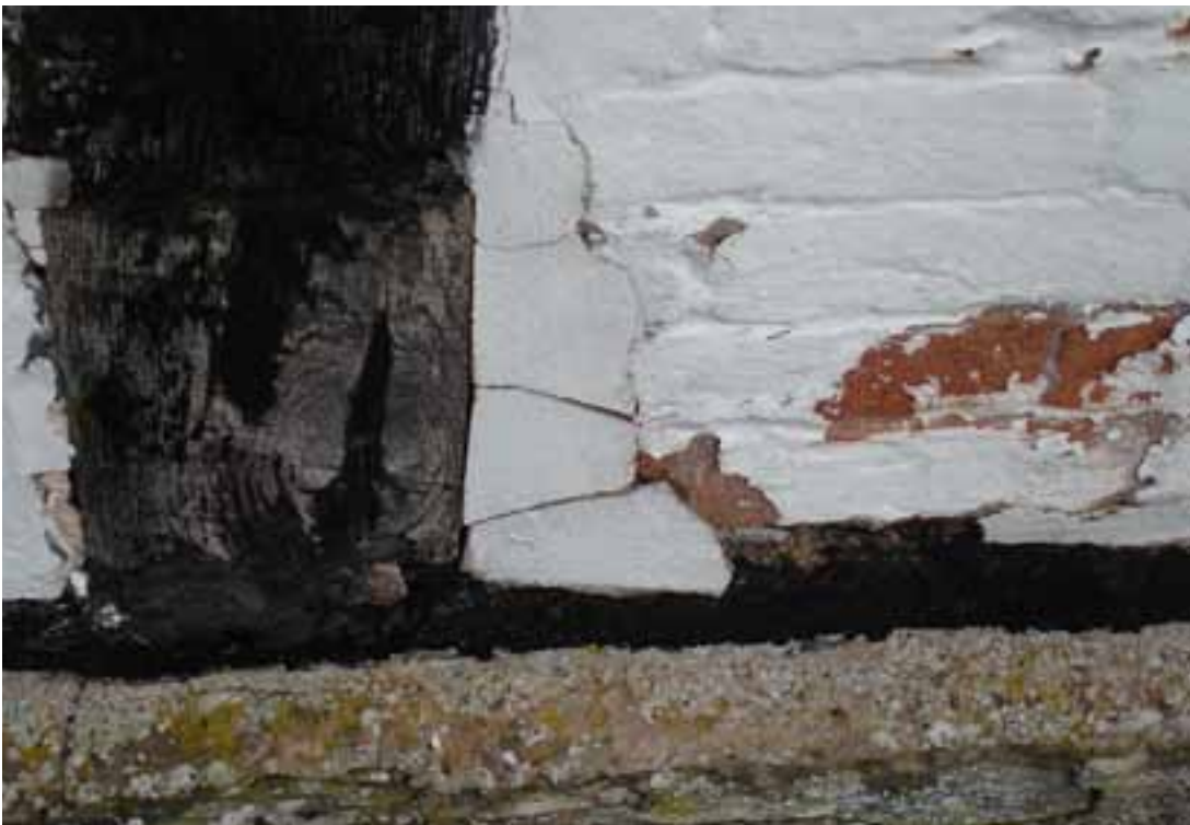
06 A hard cement mortar has been used to fill the gap at the edge of a brick panel. As the mortar is inflexible it has cracked and will trap moisture against the frame possibly leading to decay. © EH/David Pickles
