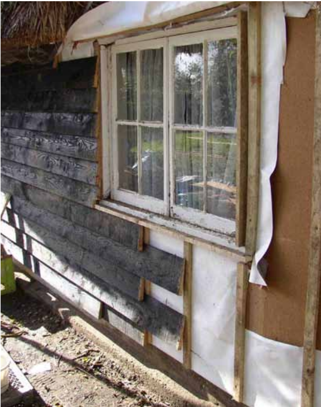
16 A vapour permeable membrane and tongue and grooved wood-fibre board has been added onto the frame below weatherboarding. © Oxley conservation
