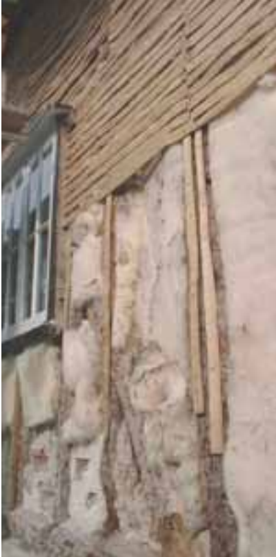
12 Timber laths being added over a frame to take an external lime render. Sheep's wool insulation has been added between the frame. © Oxley conservation
