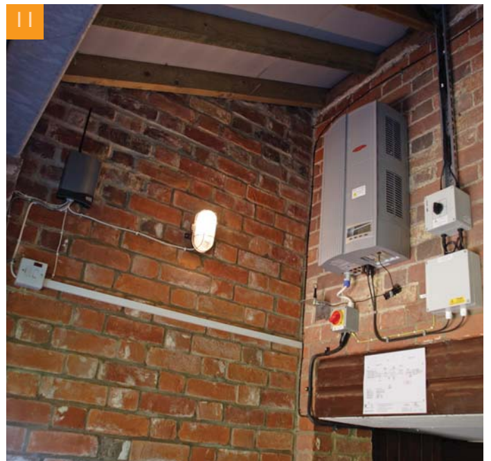
11 An installation, showing the inverter, isolator. (Photograph courtesy of Solar Century.)
