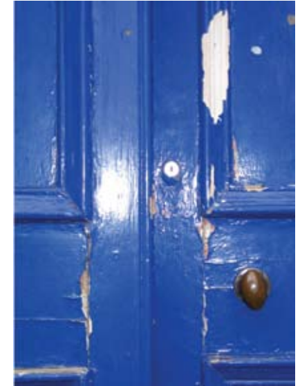
If not regularly maintained paint will begin to peel from doors leaving them vulnerable to further deterioration.
