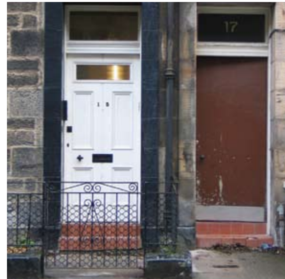
The difference between retaining a traditional door and a poor quality replacement.
