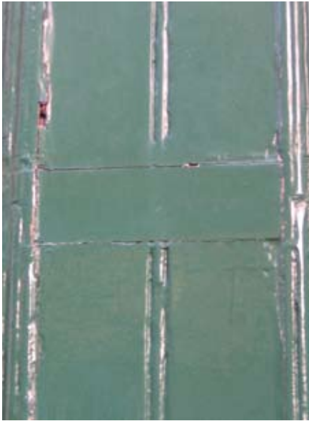
A poor quality repair where a letterbox was present.
