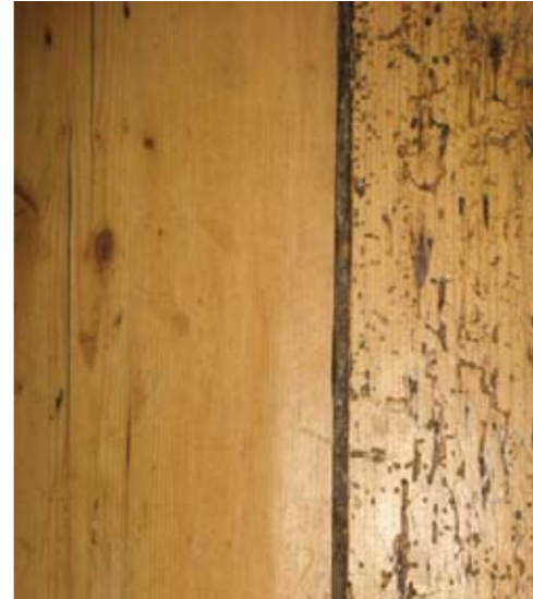
19th C flooring, showing wood beetle attack (no longer active) on the softer timber.
