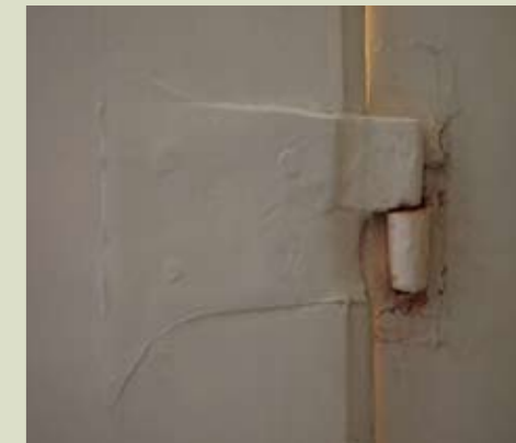
Hinged connection between secondary and outer shutter leaves and outer shutter leaf and window jamb
