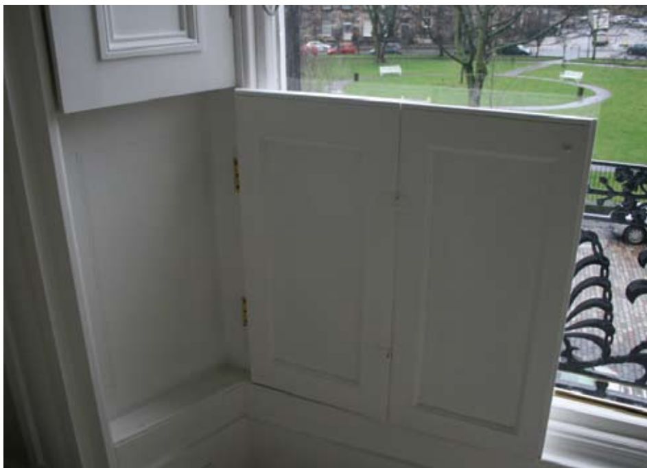
A well maintained shutter folding into recess
