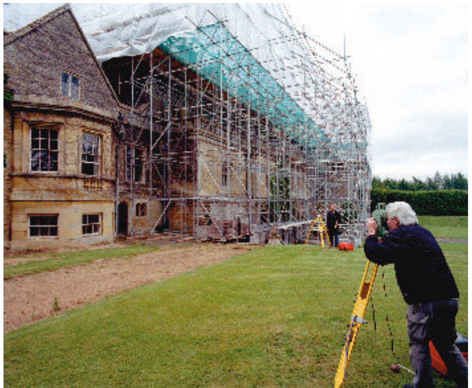
Figure 11 EDM or REDM theodolites can confer immense benefits in both time and accuracy, in surveys of large, complex or irregular buildings, although they cannot make up for poor observation or a lack of understanding. (Apethorpe Hall, Apethorpe, Northants; AA044523)
